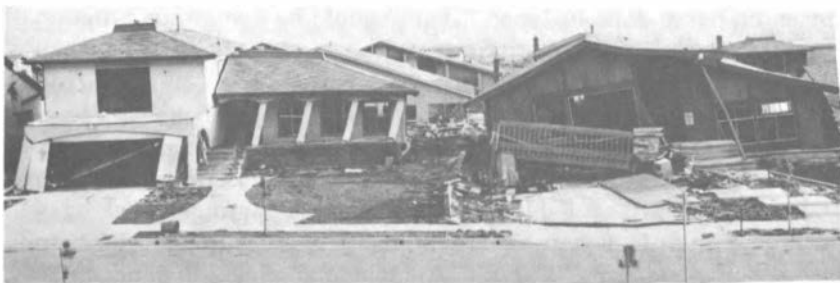
These split-level houses were damaged by the 1971 San Fernando earthquake. In this type of structure, part of the house is built above the garage, so special bracing is needed to resist seismic forces.
