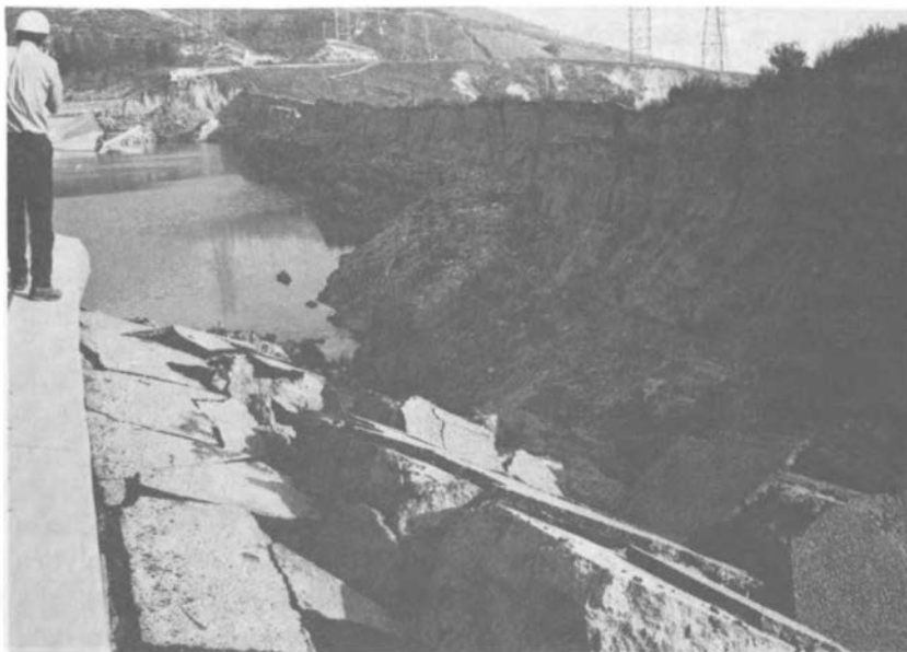
The upstream slope of the Lower San Fernando Dam slid beneath the water during the 1971 San Fernando earthquake, leaving just 4 ft of freeboard. This 140-ft-high earth dam was constructed prior to 1920 at a time when earthquake hazard was not considered.
