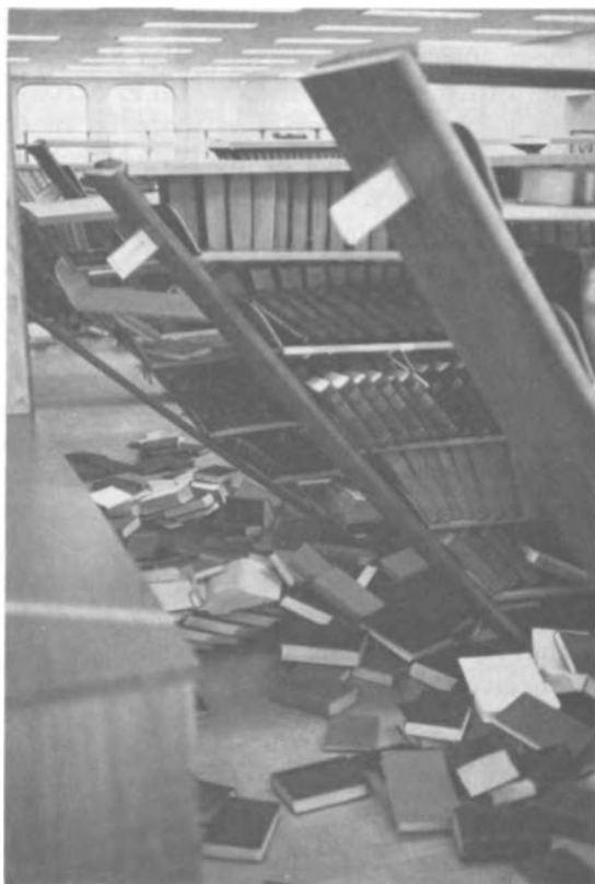
These library shelves collapsed during earthquake shaking. Equipment, bookshelves, lighting fixtures, and all other items that could be hazardous must be designed to withstand earthquake forces.
