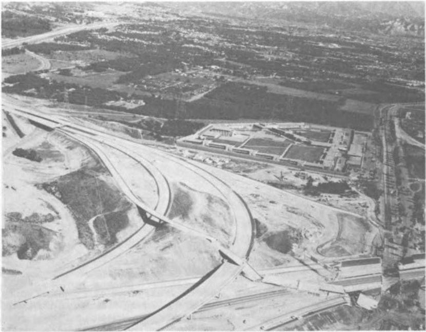
This freeway interchange bridge in Sylmar, California, collapsed during the 1971 San Fernando earthquake. In the lower right-hand corner a collapsed overpass bridge has been partly cleared away. In the center of the photograph can be seen a large new juvenile detention facility, which was so badly damaged that it was later demolished.
