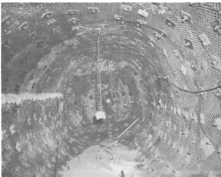
FIGURE 12 Structure with rock bolts and mesh—end-on loading, sections CR5 and CR6 (event Pile Driver).
