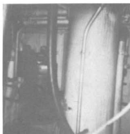
Figure 7.1.10. Generator room fire pump.
