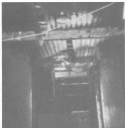
Figure 7.1.22. Overhead damaged at main vertical zone.
