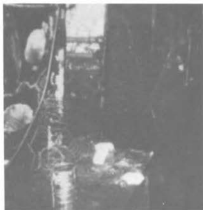
Figure 7.1.14. Hydraulic control room entrance.
