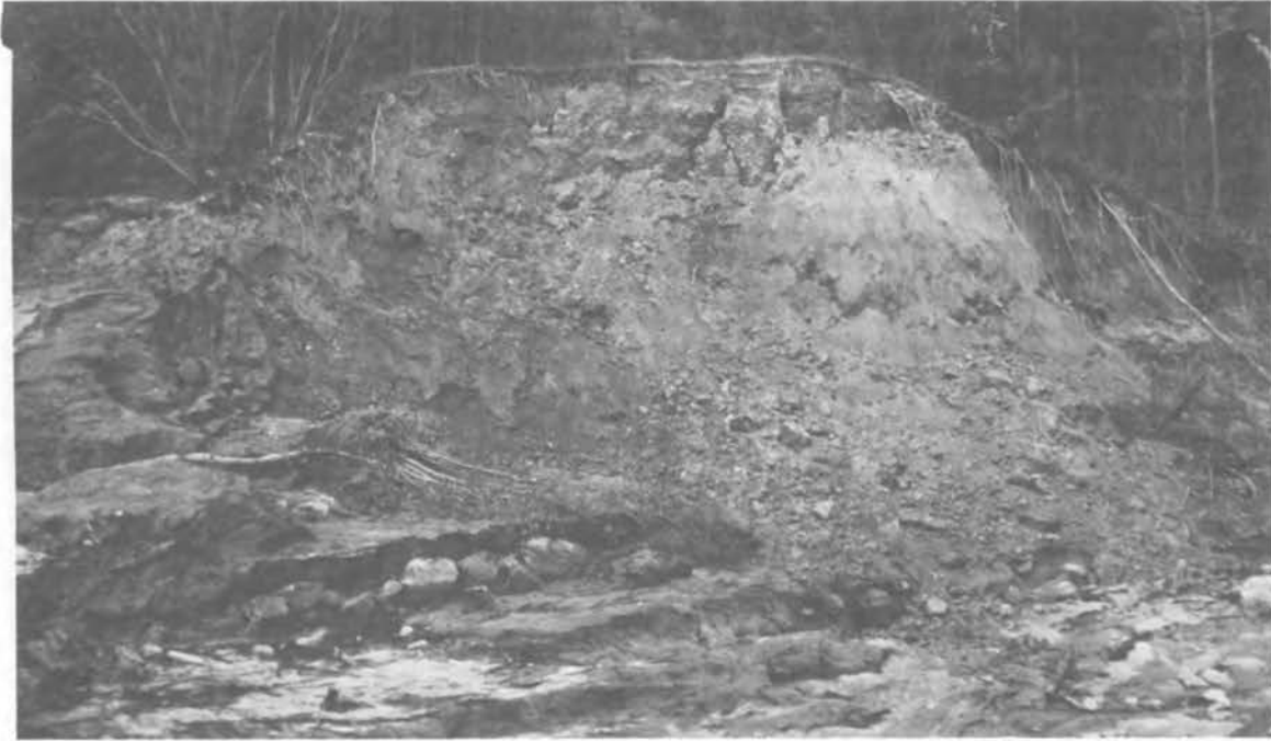
FIGURE 7 Face of breach on left side, looking north, upstream to left
