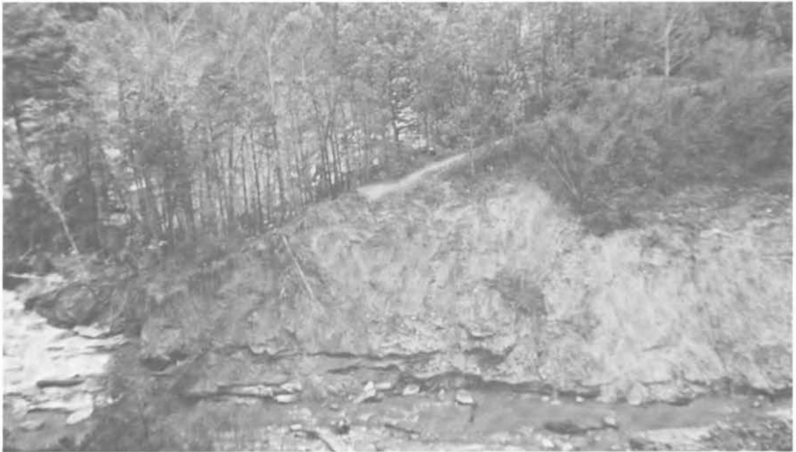
FIGURE 5 Face of breach on right abutment looking downstream
