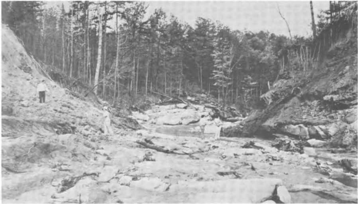
FIGURE 4a Dam looking downstream through breach
