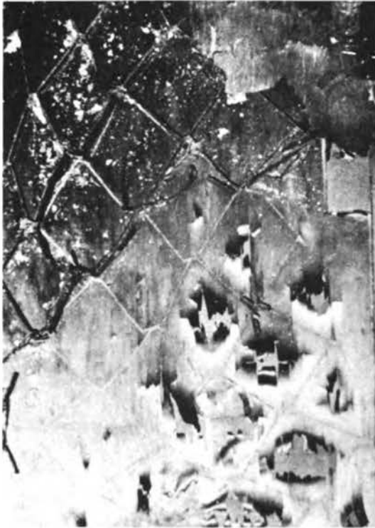
FIGURE 3. Burned exterior of hollow-core wood panel door.
