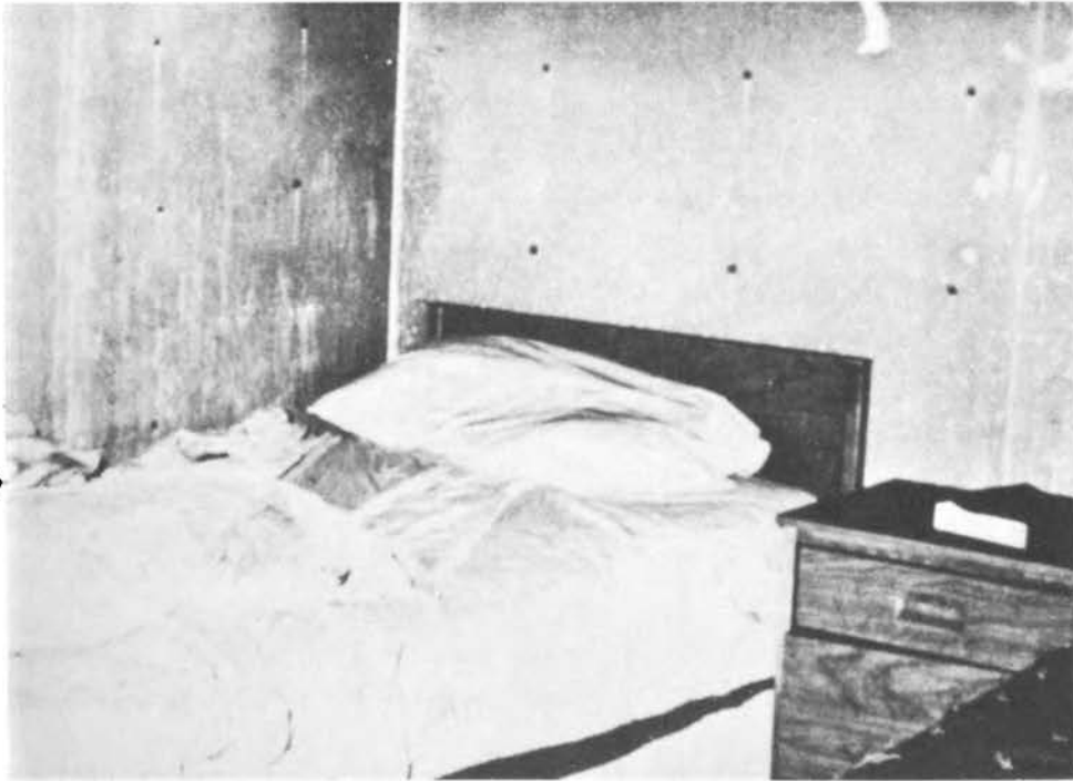
FIGURE 6. Typical smoke and soot pattern south second story bedroom.
