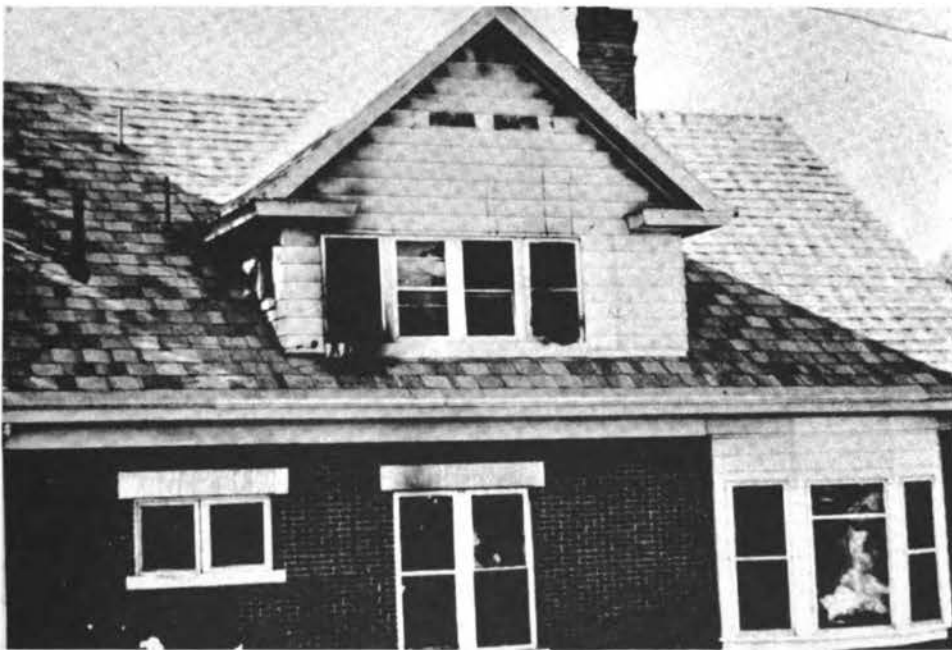
FIGURE 2. Exterior side view of the Lil-Haven Nursing Home after fire.
