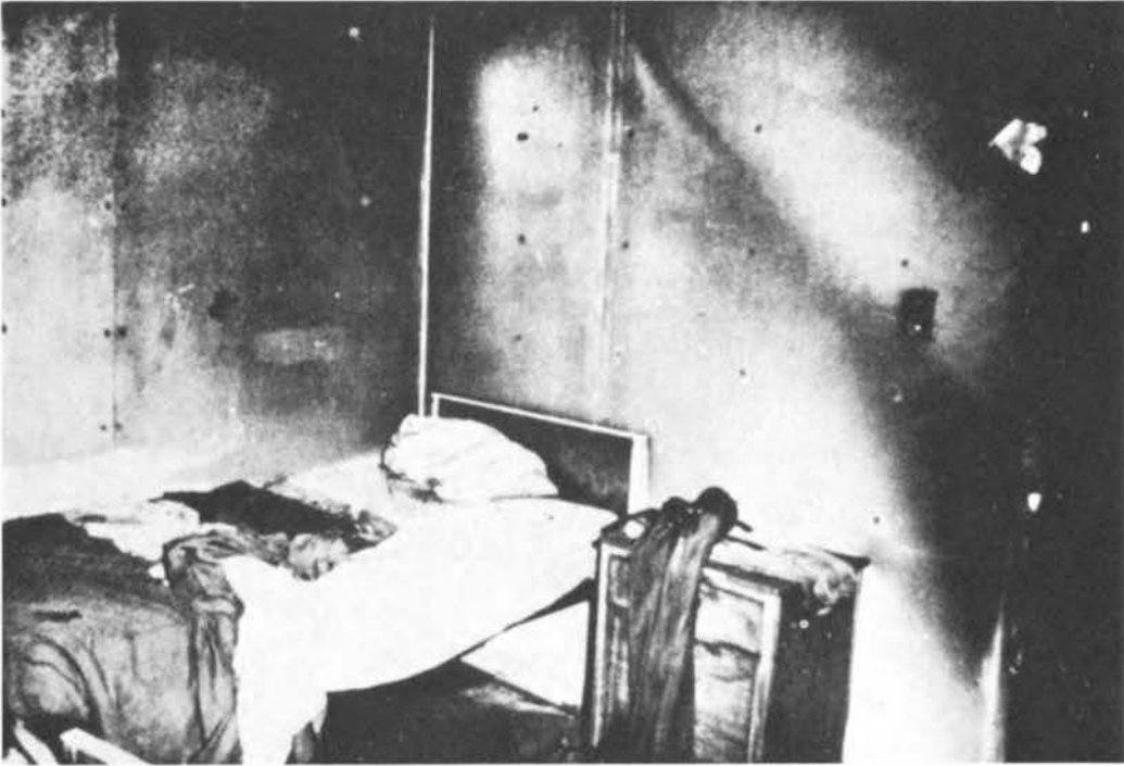
FIGURE 5. Typical smoke and soot pattern north second story bedroom.
