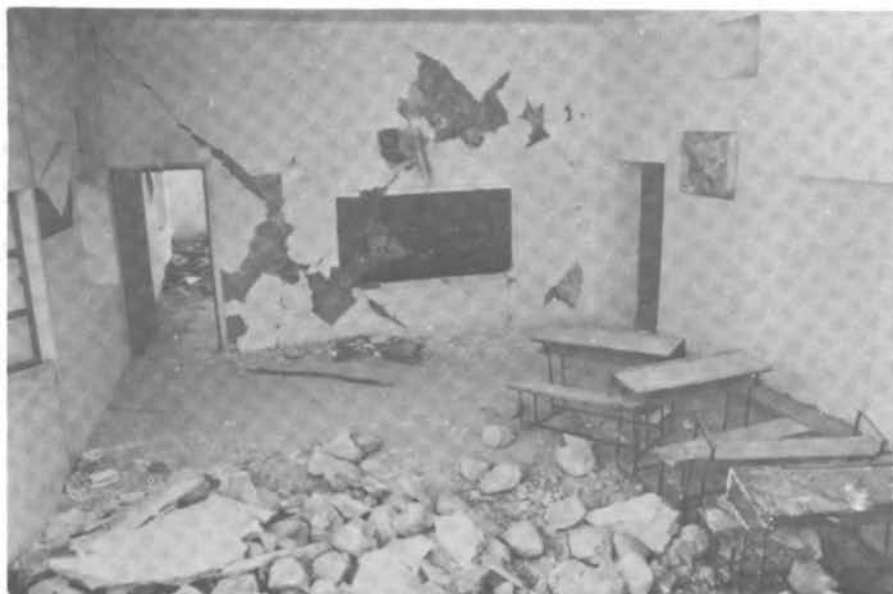
FIGURE 3.50 A View of the Cracked East-end Interior Partition Wall of the Ābe Garm School.
