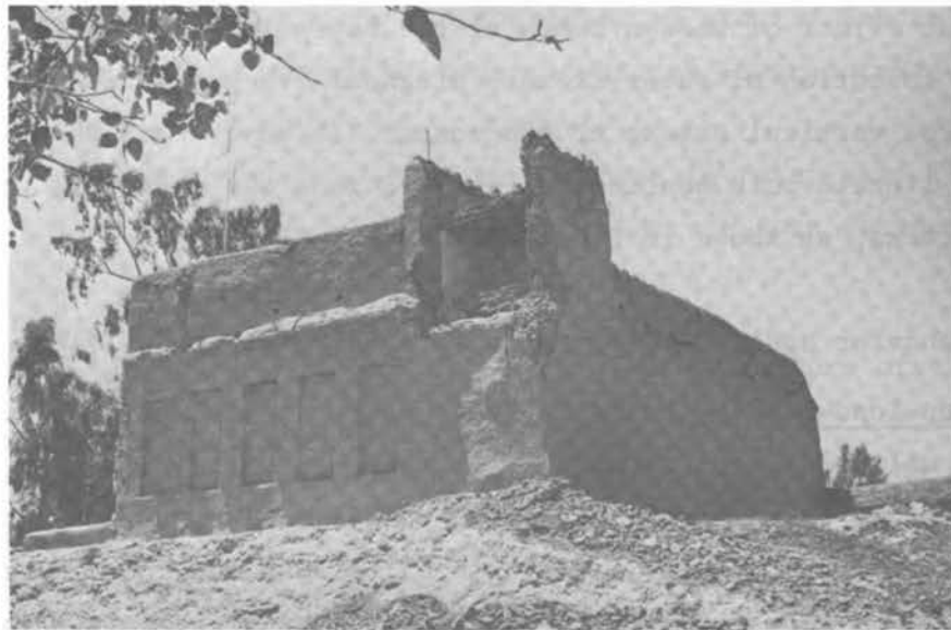
FIGURE 3.71 Collapse of One of the Upper-story Non-load-bearing Walls of the Gendarmeri (Rural Police) Station at the Village of Laghar.
