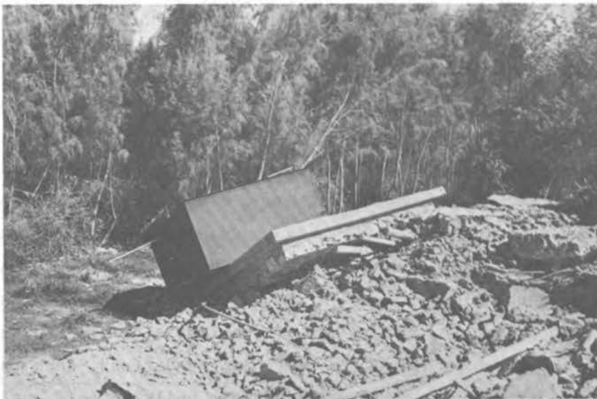
FIGURE 3.61 The Ruins of a Reinforced Concrete Slab Supported by Adobe Walls.
