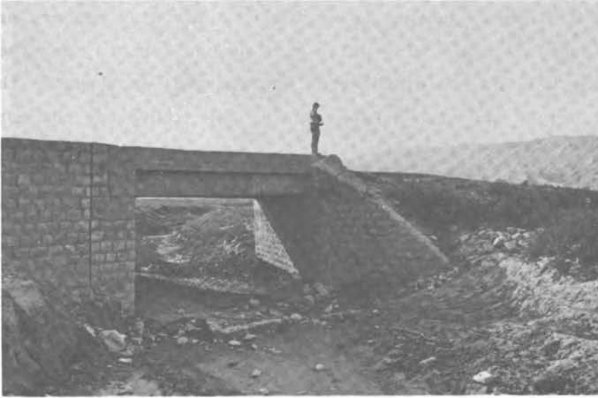
FIGURE 3.39 Failure of the Wing Wall of a Small Bridge near the Village of Khayrābād (No. 3).
