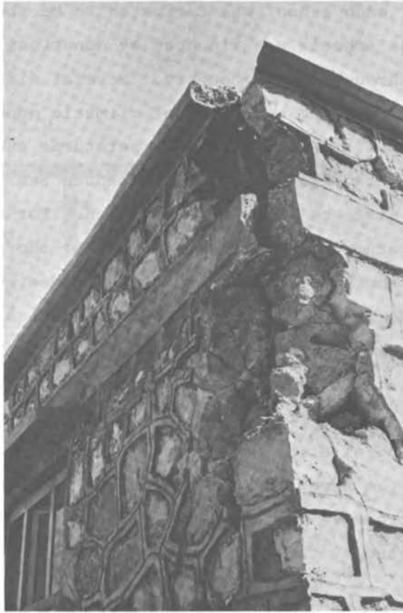
FIGURE 3.45 Failure of the Tie-beam at a Corner Due to the Lack of Corner Reinforcement.
