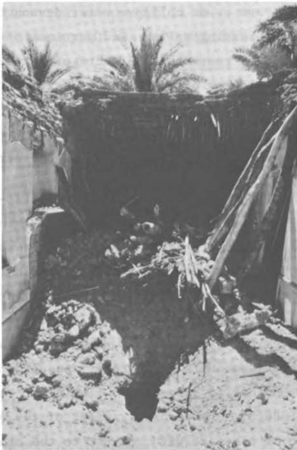
FIGURE 3.74 Typical Failure of a Roof Due to Insufficient Length of Bearing of the Timbers (Village of Deh-beh).
