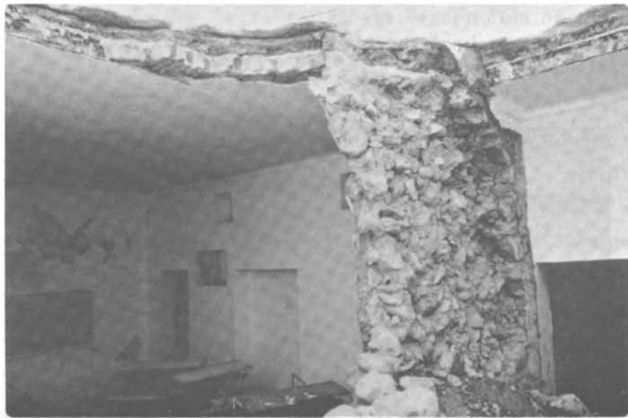
FIGURE 3.49 Interior View of the Central Classroom. Note the Mode of Failure of the Interior Load-bearing Stone Masonry Wall.
