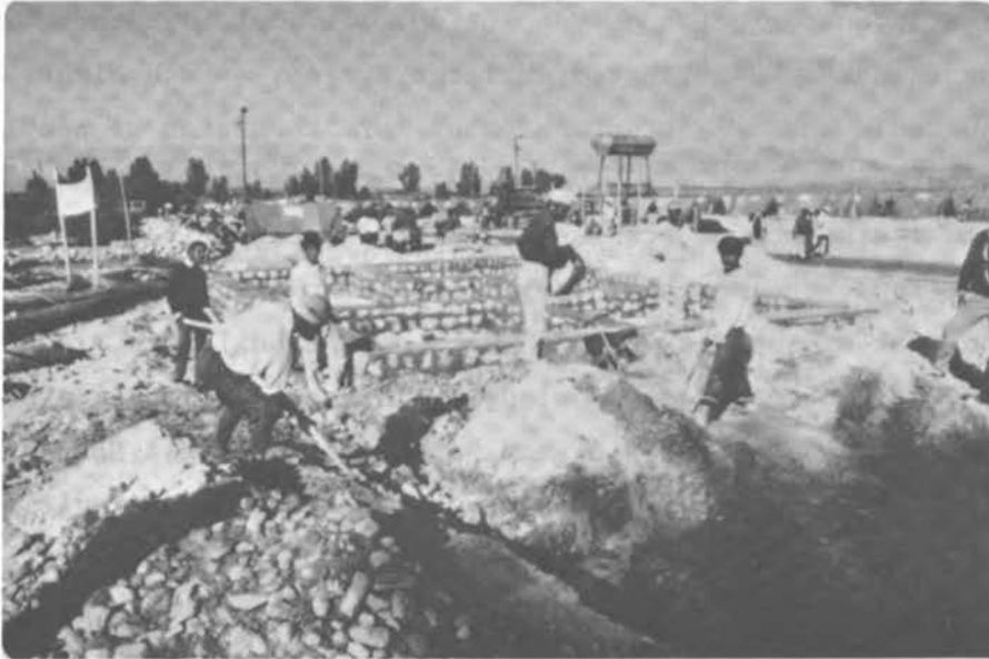
FIGURE 4.3 The Foundation of a New Structure Being Built Again with Rubble Stone.
