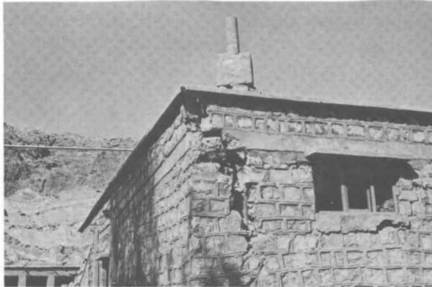
FIGURE 3.44 Failure of the Structure at the Corner Due to the Weakness in the Tie-beam and Existence of a Weak Line Along the Chimney Inside the Wall.
