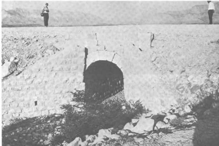
FIGURE 3.41 Damage to a Circular Culvert and its Retaining Walls near the Village of Shāhābād.
