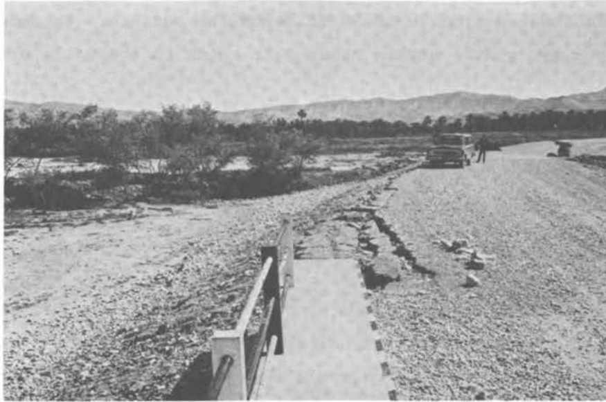
FIGURE 3.89 Damage to the Road Embankment Near the Eastern End of the Shāhābād Bridge.
