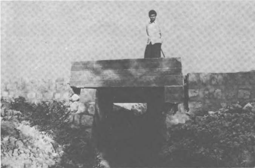
FIGURE 3.40 Failure of a Culvert near the Shāhābād Bridge.
