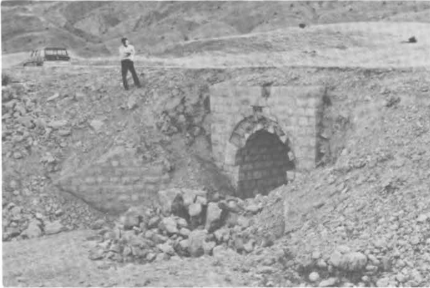
FIGURE 3.42 Damage to a Masonry Circular Culvert and its Wing Walls, near the Village of Shahabad.
