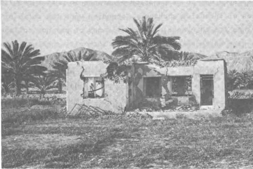
FIGURE 3.70 Typical Failure Mode and Crack Shapes of Lintels and Wall Elements.
