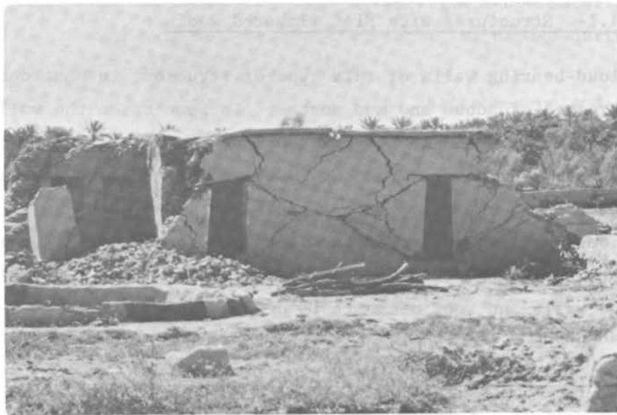
FIGURE 3.62 Typical X-shaped Shear Cracks on a Wide Adobe Wall.
