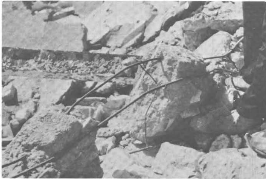
FIGURE 3.30 A Close-up View of the Destroyed Reinforced Concrete Tie-beam of the Marand School.
