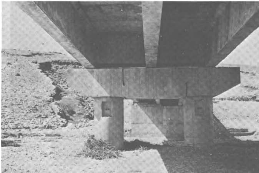
FIGURE 3.35 First Interior Support from the Eastern Abutment. The Locations of Hair Cracks are Marked.
