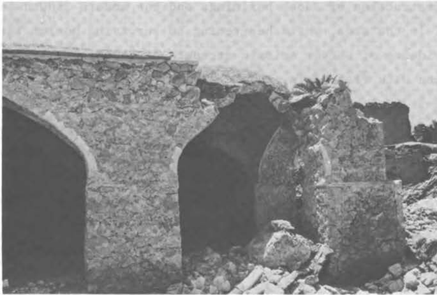
FIGURE 3.77 Damage to the Southeast Corner of the Friday Mosque of Bian.
