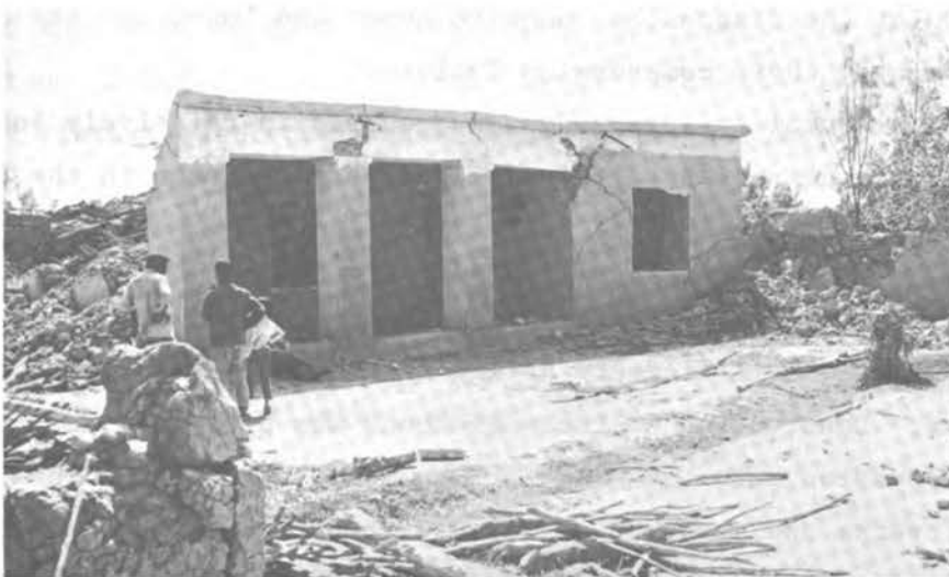
FIGURE 3.68 Shear and Flexural Cracks in the Load-bearing Wall Elements and Lintels of an Adobe Building.
